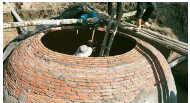
RENEWABLE ENERGY - BIOGAS
