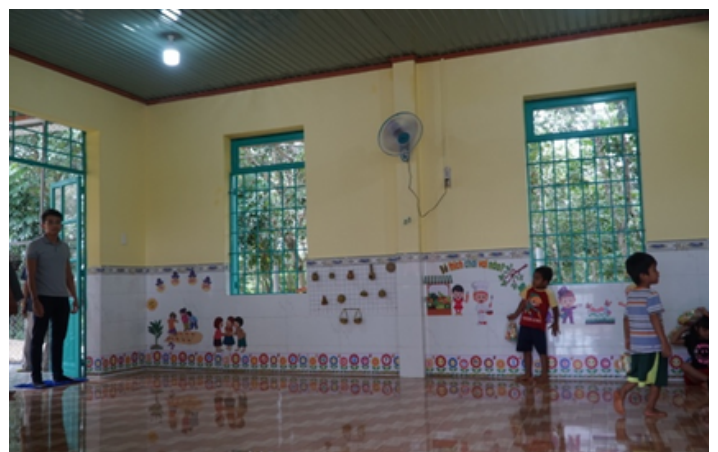
Wall was in proper paint. Newly tiled classroom background. The inox window was installed. The new light system and electric system was installed
